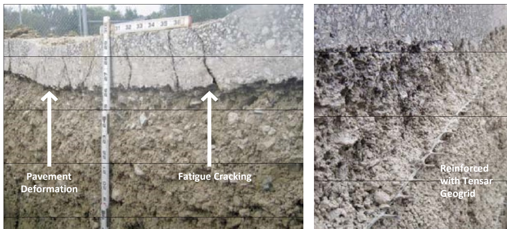
FIGURE 13 The post-trafficked trench section (on the right) reveals a dramatic reduction in asphalt and aggregate deformation due to the inclusion of a Tensor Geogrid when compared to the unreinforced section pictured on the left.
