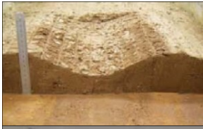
Subgrade rutting with Tensar BX Geogrid
