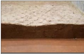
Subgrade rutting with Tensar TriAx Geogrid
