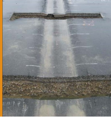
Excavations through each test section reveal the significant influence of the Tensor® Geogrid reinforcement.
